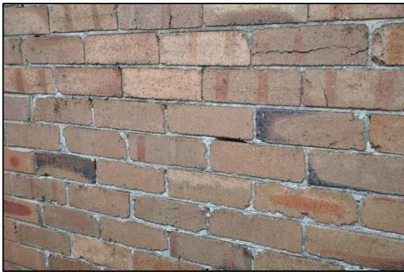
Figure 22. Close up view of original brickwork showing erosion of mortar.
