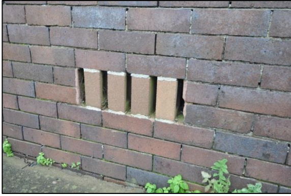
Figure 19. Unsympathetic ad-hoc ventilation at sub floor level.
